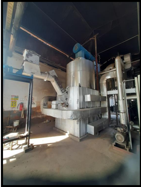
Thermic fluid heater
